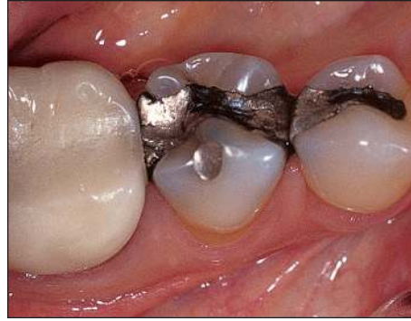
Fig 11-10 Defective mesio-occlusodistal (MOD) amalgam restoration in the mandibular second premolar. Excessive width and need for cusp replacement precludes this amalgam restoration from being replaced with resin composite. A discolored fracture line and recurrent caries running from the MOD amalgam to the amalgam in the facial cusp tip would necessitate functional cusp coverage with the replacement restoration.
